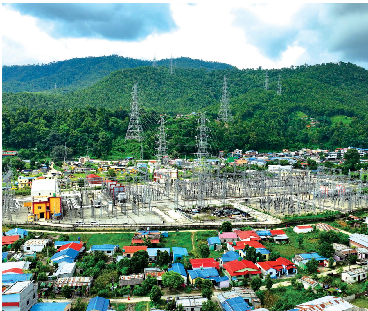
Overview of the Hetauda 400KV Substation Supporting Cross-border and Regional Power Transmission.
