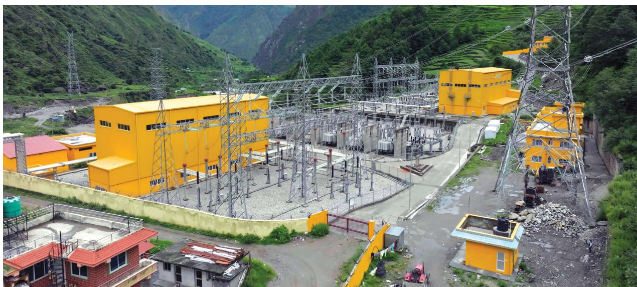
Chilime Substation and Transmission Hub, Rasuwa
