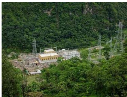
220/132/33 kV, 200 MVA Rahughat GIS Substation
