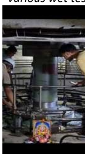
Spinning Test of Unit-1 and Monitoring Temperature and Vibration
