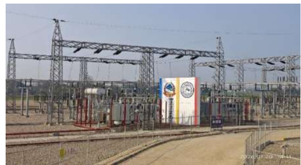
Switchyard of AIS Substation
