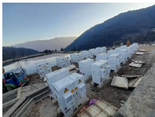
BESS Installation in Jumla
