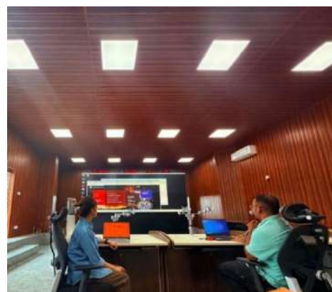
Master Control Center- Pokhara
