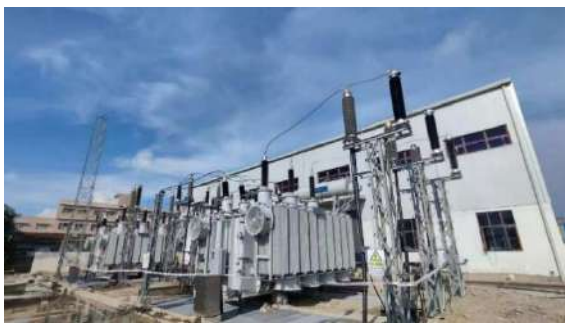
Transformer and GIS Substation
