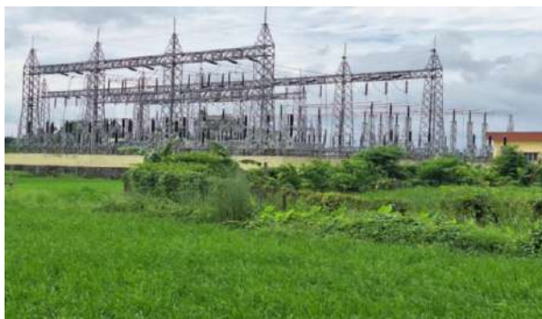
132 kV Switchyard area for Keraun 132/33 kV Substation Work
