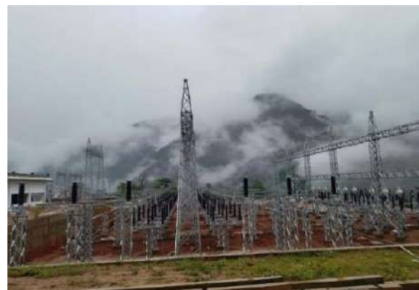
Overall View of Khungri Substation
