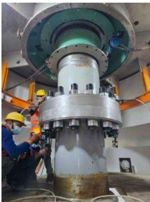
Unit-1 Generator and Intermediate Shaft Coupling
