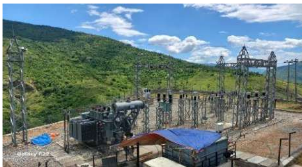
33/11 kV, 6/8 MVA Tumbewa, Panchthar Substation Handover to Panchathar DCS
