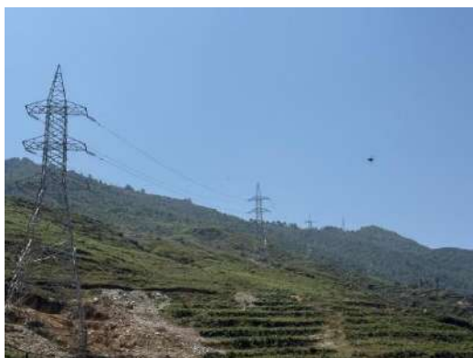
Balefi Corridor transmission line
