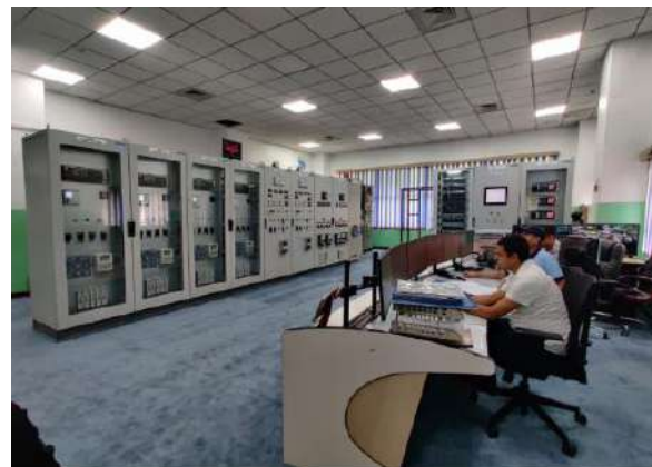
Control Room of Kulekhani I HPS
