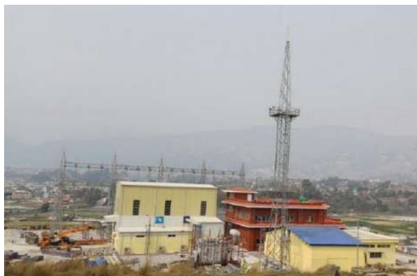
132/11 kV Changunarayan Gas Insulated Substation
