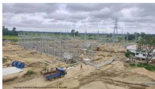
Balganga Substation switchyard
