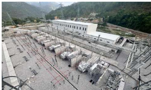
400 kV GIS Building and Transformer Banks at 400/220 kV 630MVA New Khimti Substation
