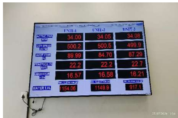
Live SCADA control display showing full 102 MW capacity generation operating smoothly across all three generating units (~34 MW each)
