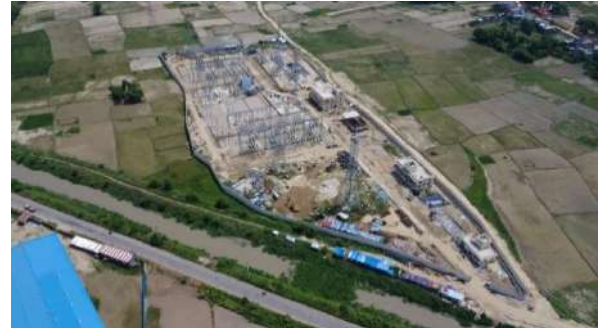
Aerial View of Prasauni 132/33/11kV AIS Substation
