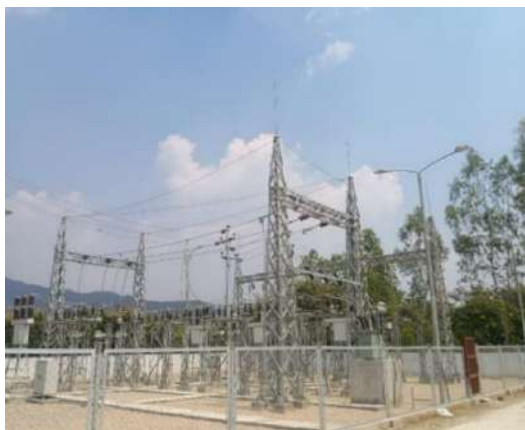
33/11 kV Siraha Substation
