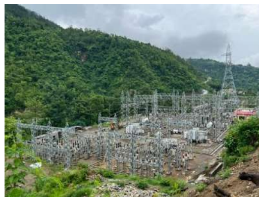
Switchyard at Ridi 132/33/11 KV Substation
