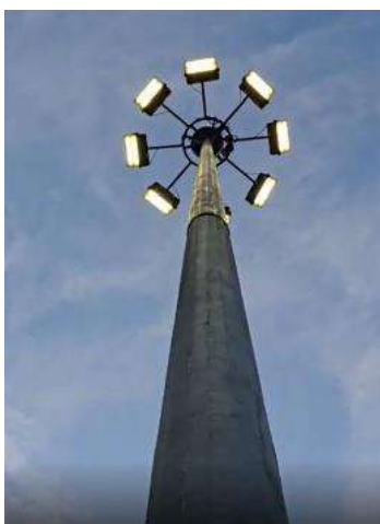
High Mast Street Light
