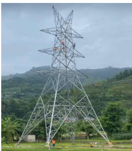
220 kV Transmission Line Tower
