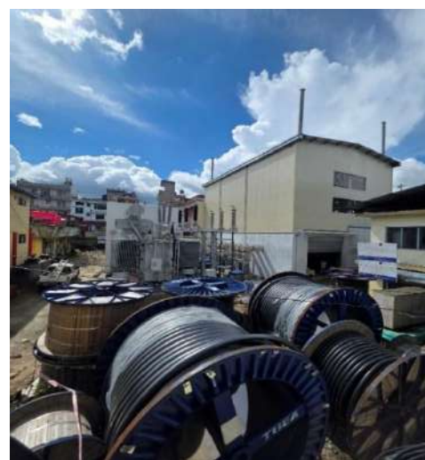
Imported XLPE Cable at Patan SS
